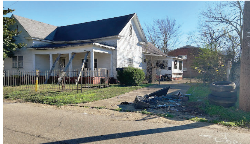
This dilapidated home is located in one of Columbus’ “Gateways” (a high-traffic, high visibility area) and was reported on SeeClickFix in June 2020.
